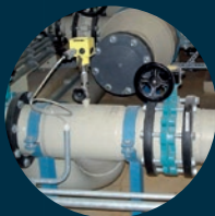
Flue Gas Desulfurization
