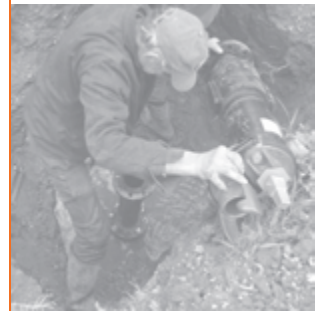
Hydrants and Connections
