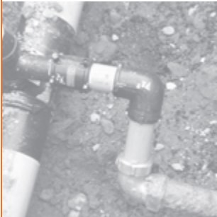
House Connections & Service Lines
