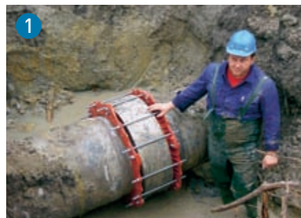
Repair of leaking joints under pressure. WAL/V leak clamps provide a dependable repair solution.
