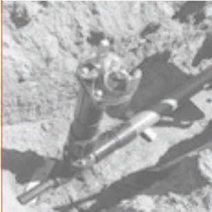
Hydrants and Connections
