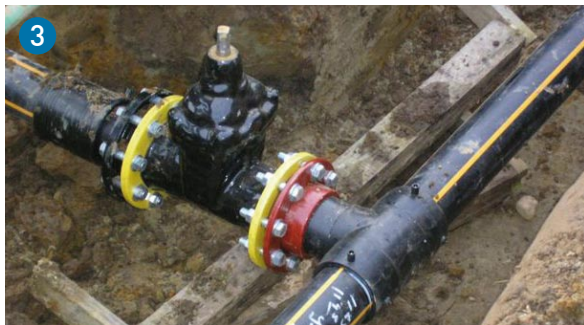
Simple installation technology: PE branch off with the Draw Lock flange connection
